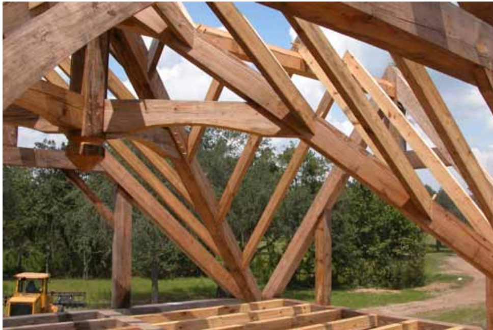
Unequal pitched joined timber frame valley system built using the Chappell Universal Square system. Main pitch 15/12, secondary pitch 9/12.
